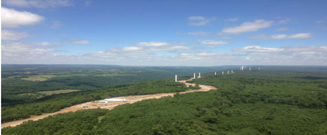
Natural gas pipelines construction concurrently with wind turbine construction along a ridge in the Marcellus.
